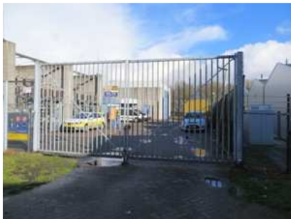
50/10 kV station (Transformatorstation)
